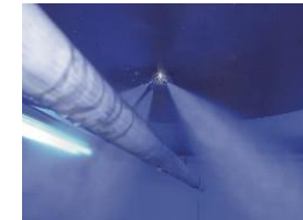
Fogtec Fire-Fighting System
